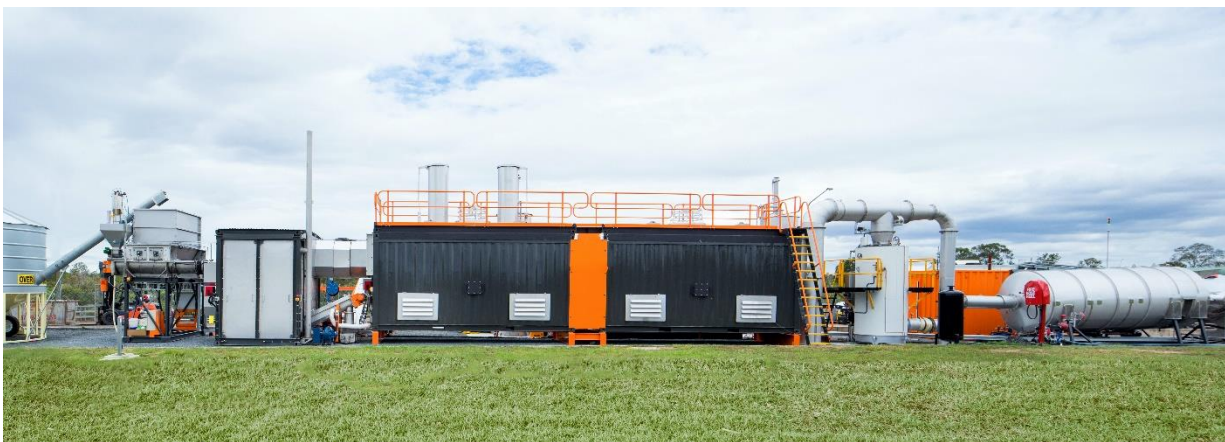
Demonstration plant located at Loganholme wastewater treatment plant, showing full processing system. Image courtesy of Pyrocal.
