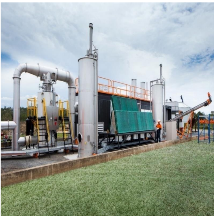
Demonstration plant located at Loganholme wastewater treatment plant, showing heat recovery system. Heat recovery unit and biosolids feed equipment are visible in the background. Image courtesy of Pyrocal.
