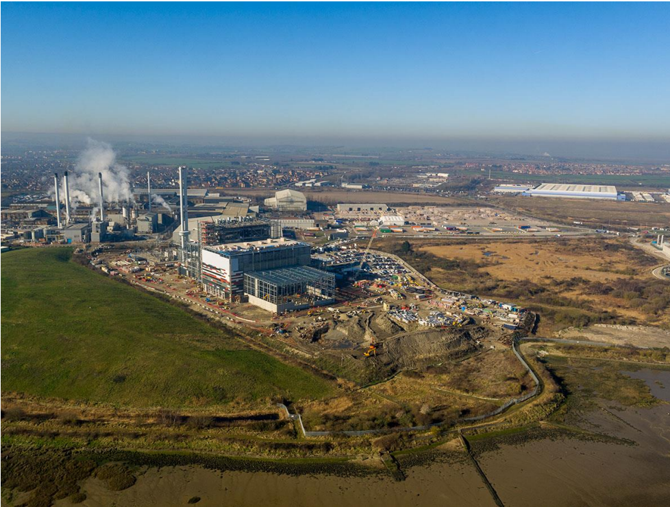
Facility under construction in 2019, with the DS Smith paper mill visible in the background. Image published by Wheelabrator Technologies
