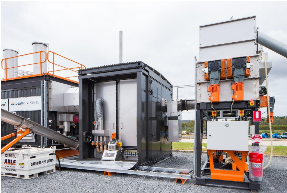
Demonstration plant located at Loganholme wastewater treatment plant, showing the hearth unit where biosolids are thermally treated. Image courtesy of Pyrocal
